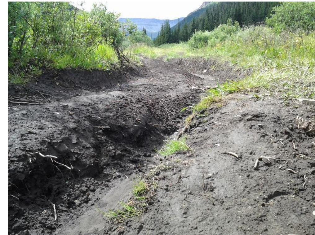
CAN damage site Taken 2017-07-24 Severity: 5 L: 72m, W: 3m, D: 55cm
